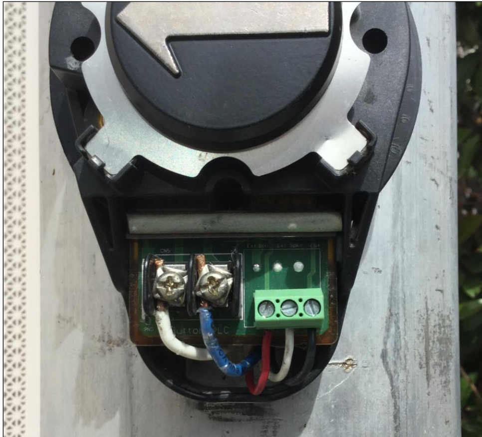
Pole-mounted iN3 PBS
