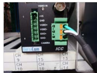
AC Power Cord Plug Installed
