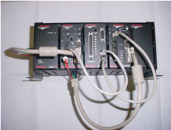
Access Module in VRack4 with Hookups
