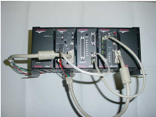
eAccess Module in VRack4 with Hookups
